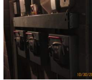
Figure E11: Disconnect Switches in Typ. Mech. Room
