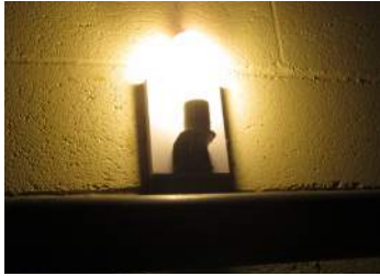
Figure E12: Typ. CFL Light Bulb in Stairwell
