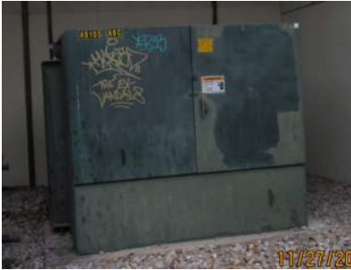
Figure E1: Existing Utility Transformer
