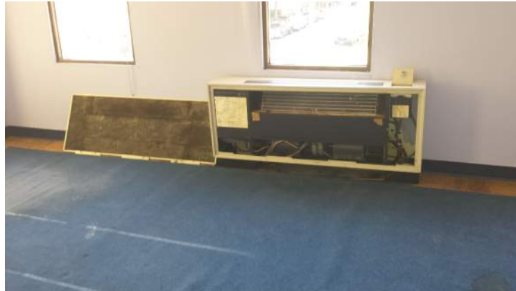
Figure M6: Existing Perimeter WSHP Console Unit
