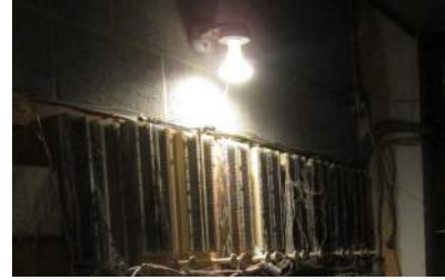
Figure E13: Typ. CFL Light Bulb in Mech. Room
