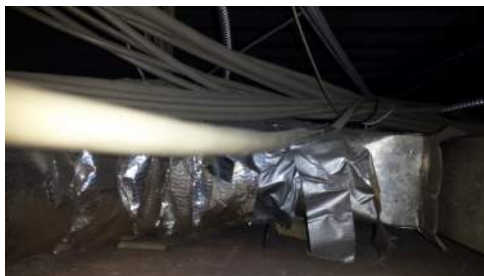
Figure M7: Poorly sealed ductwork
