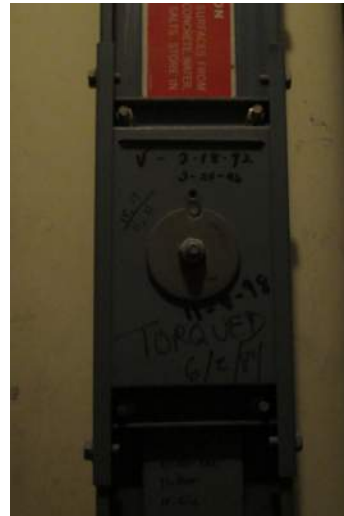
Figure E5: 400 amp Buss Risers
