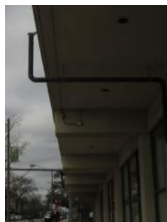
Figure E16: Exterior Lights in Canopy
