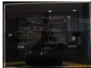
Figure E21: Fire Alarm Annunciator
