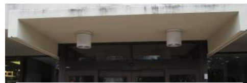
Figure E17: Exterior Light in Entrance Canopy
