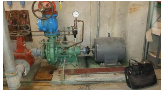
Figure P2: Domestic Water Booster Pump.
