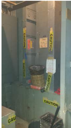
Figure E4: 2000 amp Buss Risers
