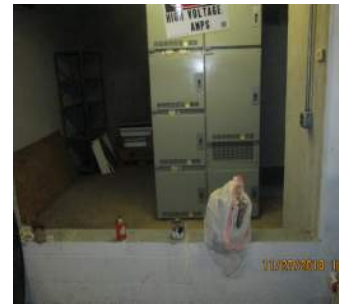
Figure E3: Existing Switchgear
