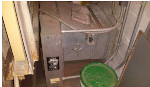
Figure M4: OA Duct in a Central Mechanical Room
