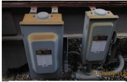
Figure E10: Disconnect Switches of Roof
