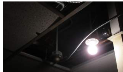
Figure E15: Typ. CFL Light Bulb in Elec. Room
