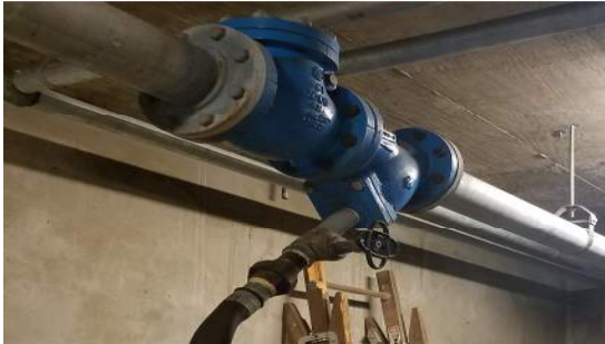
Figure P1: Existing Strainer and Check Valve Assembly.
