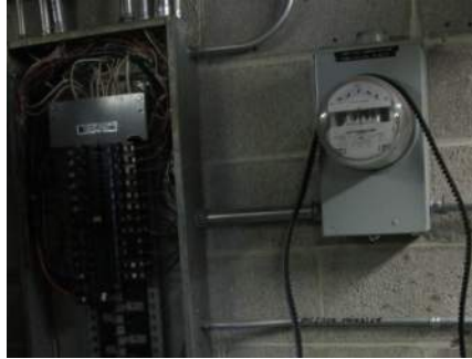
Figure E8: Sub-meter for Antenna
