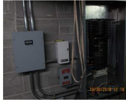
Figure E9: Sub-meter for Signage
