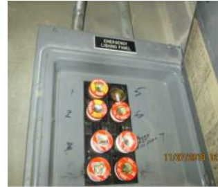
Figure E19: Emergency Light Panel
