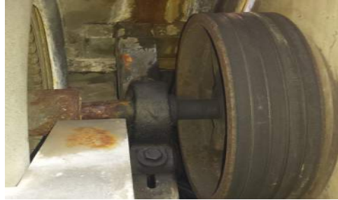
Figure M2: Corroding Fan Drive Shaft
