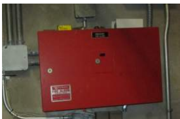
Figure E20: Fire Alarm Control Panel
